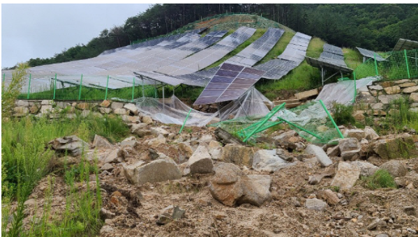
Fig. 1. Slope failure in solar power plant region (Cheorwon-gun, Gangwon province, 2020)
